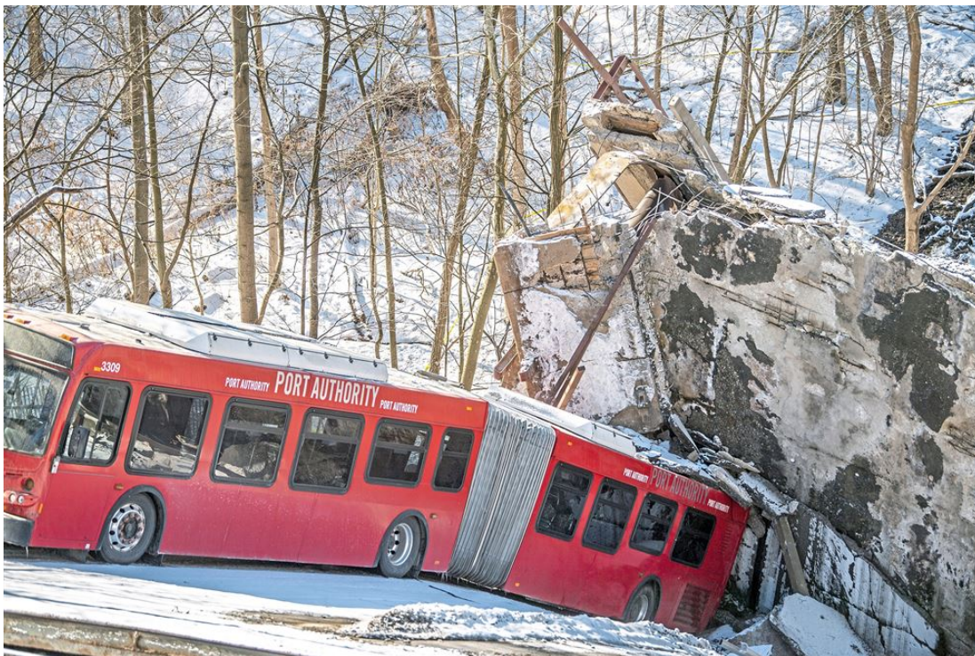
A Port Authority bus is seen in the wreckage of the collapsed Fern Hollow Bridge, Saturday, Jan. 29, 2022, in Frick Park.
